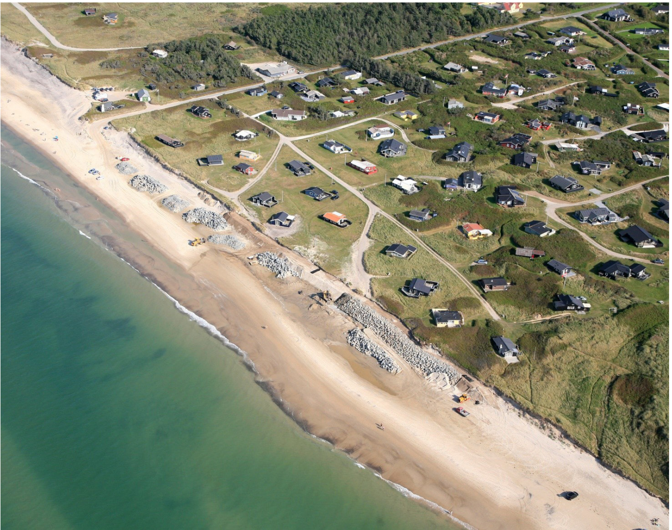
Figure 5.3: Construction of the revetment. Photo is taken on the 13th of September 2016. Notice how additional sediment has been placed behind the revetment.
